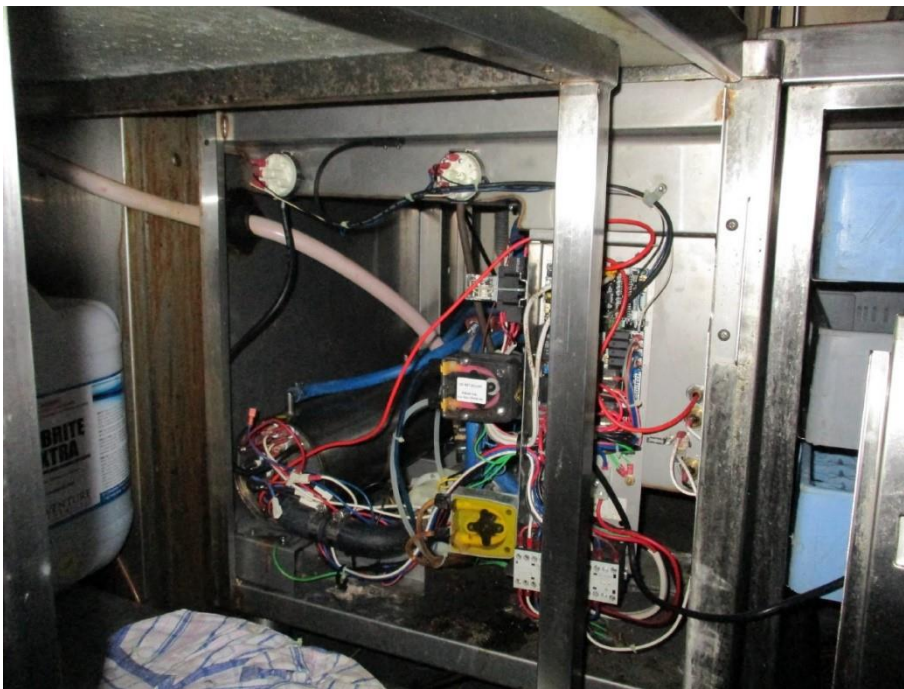
Photograph 1: The commercial dishwasher wiring and control area (3 phase supplied, covers removed)
